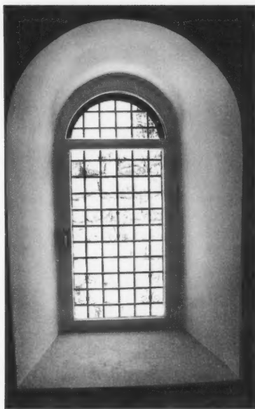
The view through a four-foot-thick, earth-filled wall at the renovated administrative annex.
